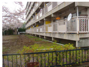
(b) 地盤沈下状況[手前側が沈下]
