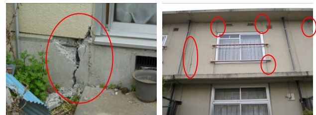
(c)基礎の破壊
